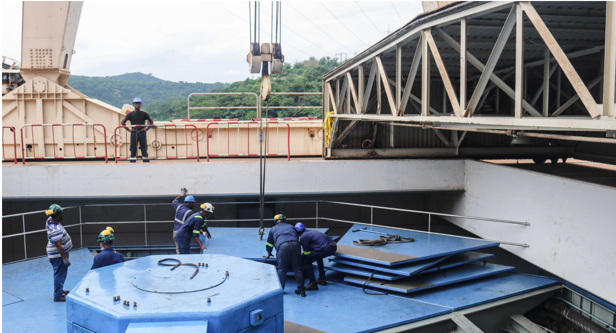
The maintenance on unit four is critical in improving its reliability and availability.
