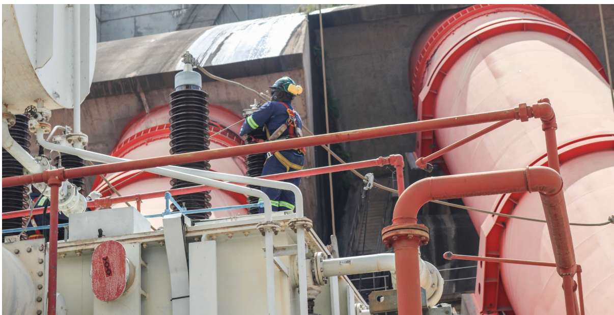
Engineers work hard to ensure high efficiency and productivity at the Akosombo plant.
