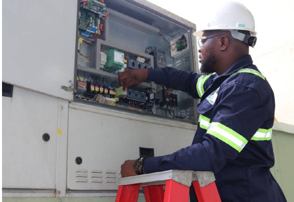
The new AC control circuit is a stand-alone panel from the old one.
